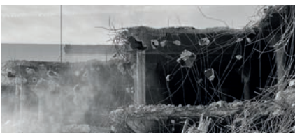
Sears, one of the oldest shopping malls in Six Corners, was deconstructed (11:01, September 30, 2021)
